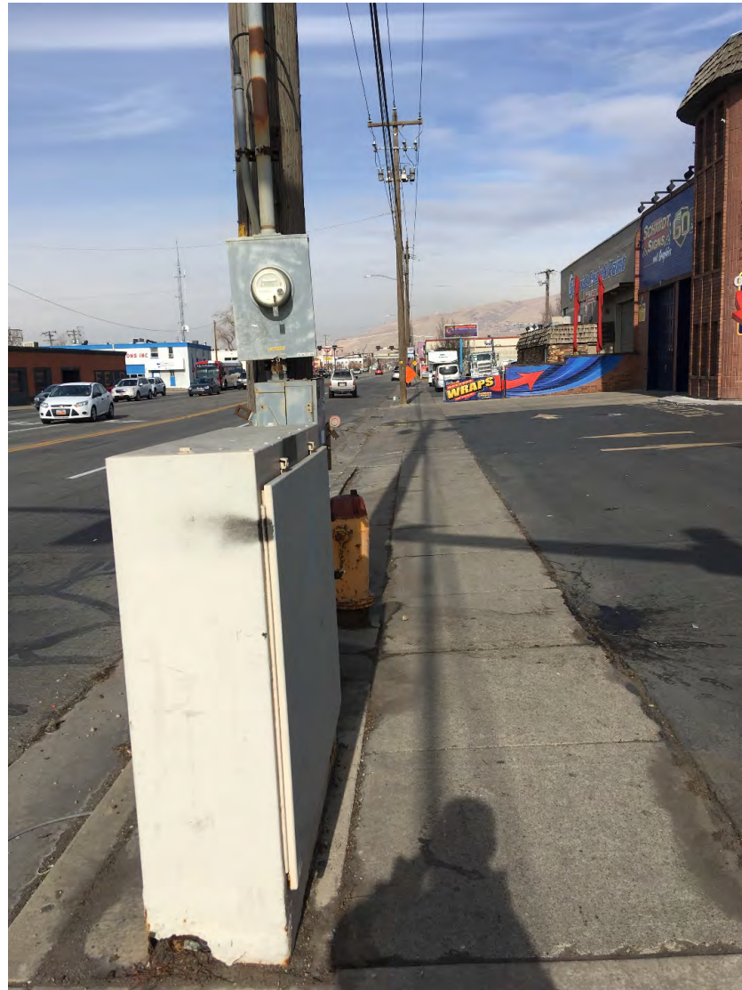
Figure 28 - Poor Sidewalk Conditions along 300 West
